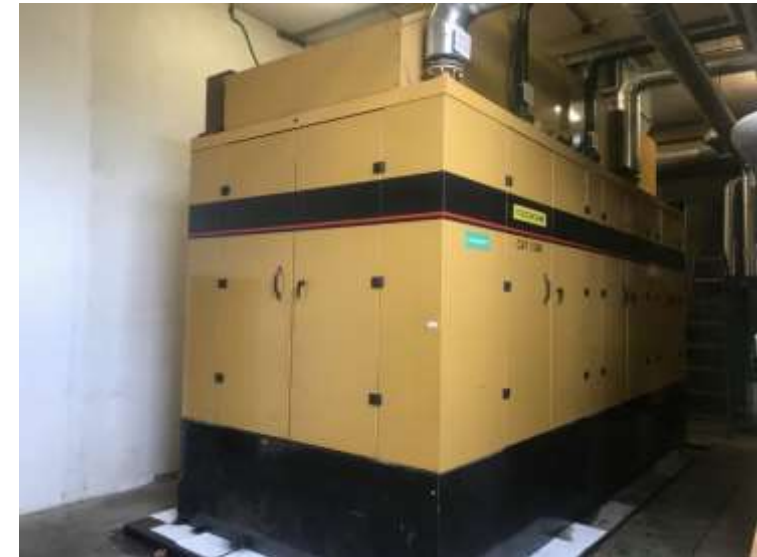
The G3516 Caterpillar type natural gas internal combustion engine
