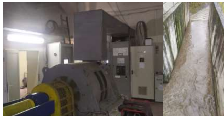
Micro-hydropower plant on the river Barnar – the electrical generator, the calming and escape channel
