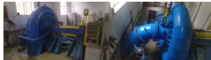
Micro-hydropower plant on the river Barnar – Francis turbine details; water discharge from the turbine
