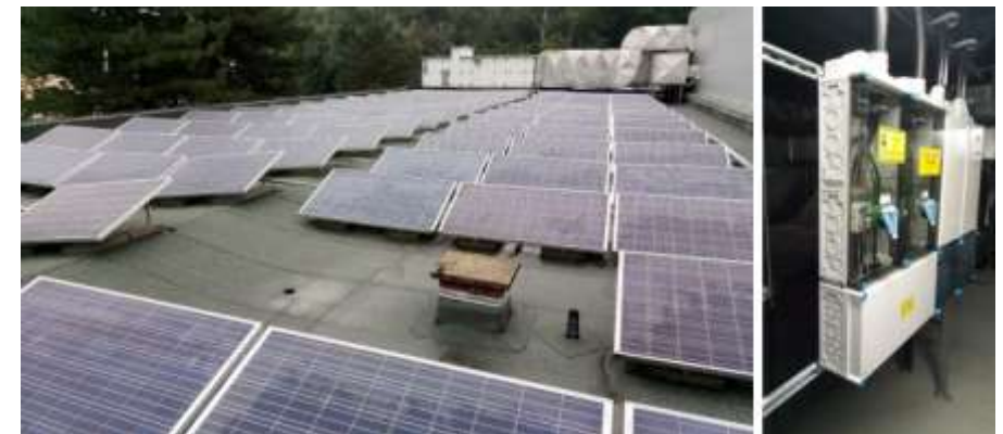
Part of the PV installation on the roof of Building B and some of the switch boxes and inverters
