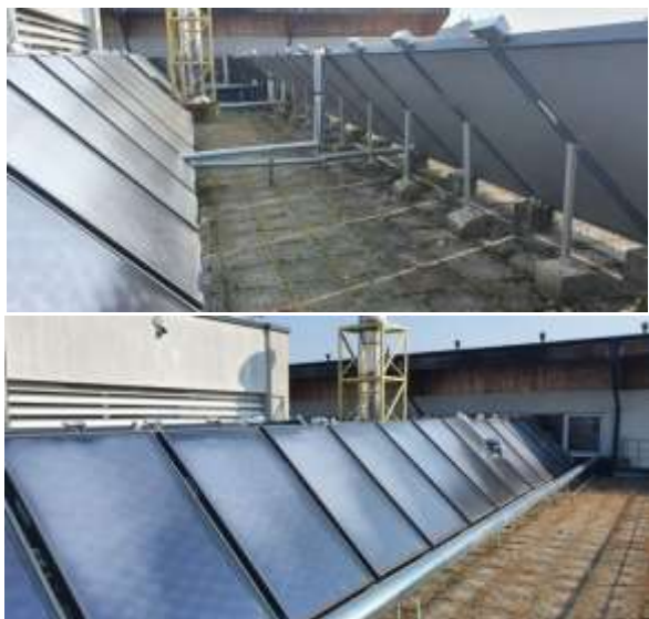
Solar thermal power plant. General view of solar collectors
