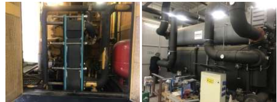
The heat exchanger of engine and the absorption chiller
