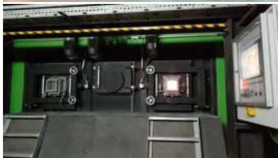
Biomass thermal power plant. Suceava municipality.
